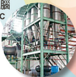
粉粒體配料/包裝機 Packing & Batching Control system
